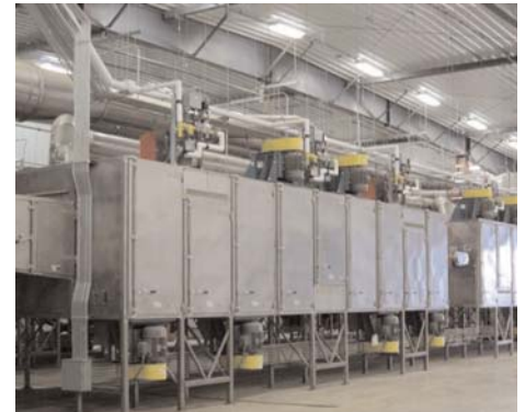
Pictured above: One of two 110' long custom designed continuous flow bed dryers.
